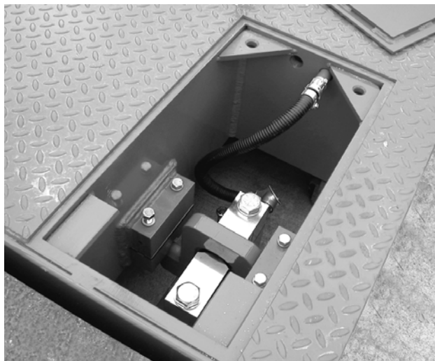
Figure 4-4. Top View of Load Cell Access Area
